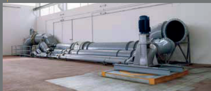
Sala prove Testing Room
